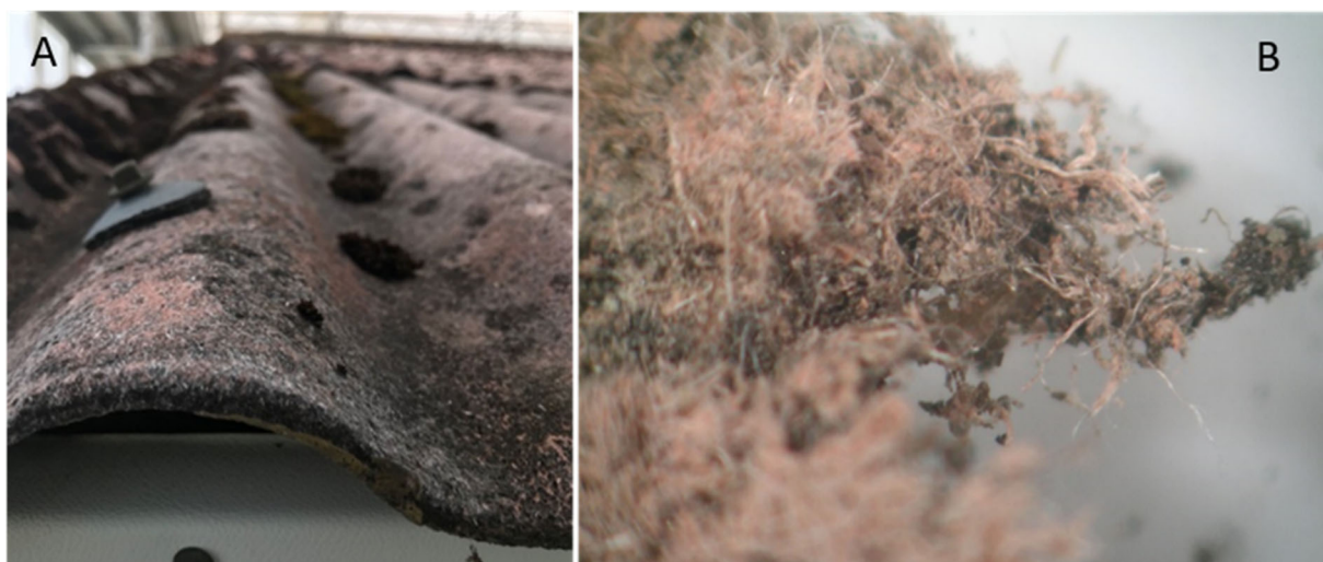
Figure 2. (A) Corrugated asbestos cement covered by moss.( B) Moss and asbestos fibers in a light microscope to the right.
